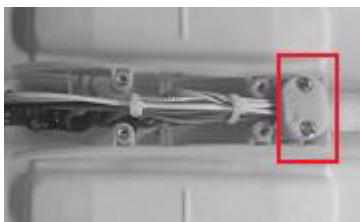
Figure 3-6 Screws in cable clamp
