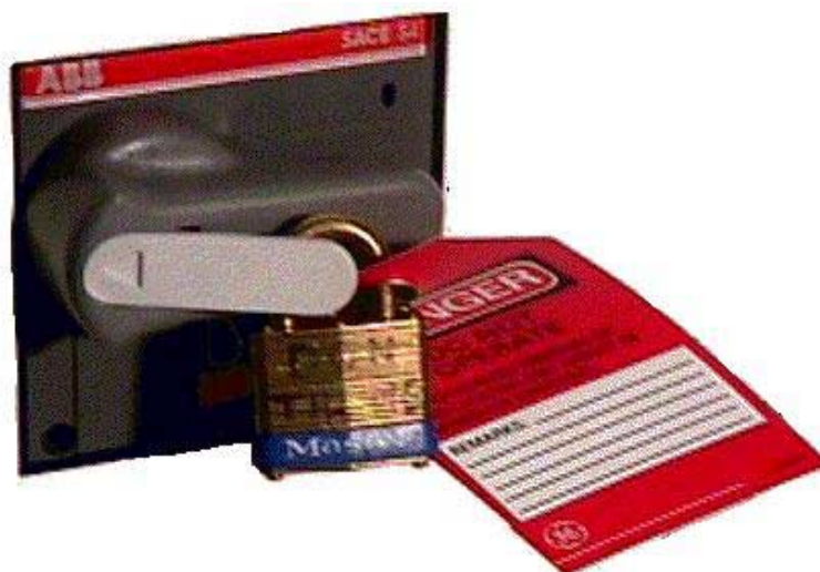
PDU MAIN INPUT CIRCUIT BREAKER LOCKED AND TAGGED OUT ILLUSTRATION 8-8
