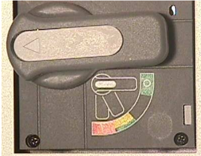
MAIN INPUT BREAKER IN THE OFF POSITION ILLUSTRATION 8-3
