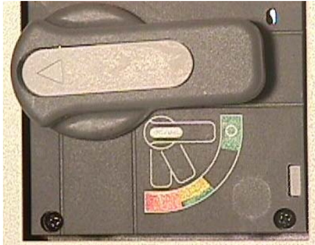
MAIN INPUT BREAKER IN THE OFF POSITION ILLUSTRATION 1-2
