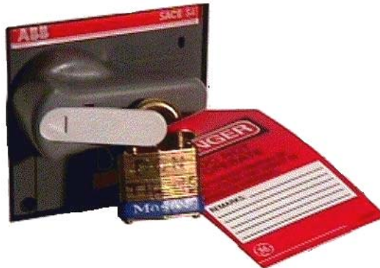
PDU MAIN INPUT CIRCUIT BREAKER LOCKED AND TAGGED OUT ILLUSTRATION 1-3
