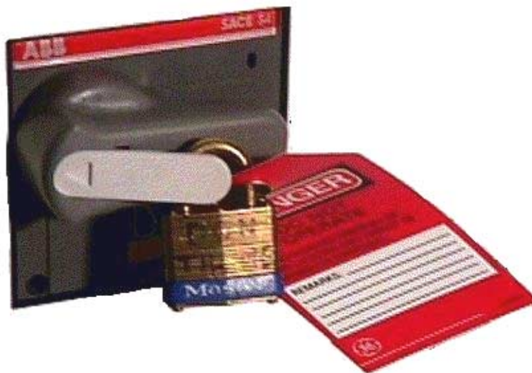
PDU MAIN INPUT CIRCUIT BREAKER LOCKED AND TAGGED OUT ILLUSTRATION 8-4
