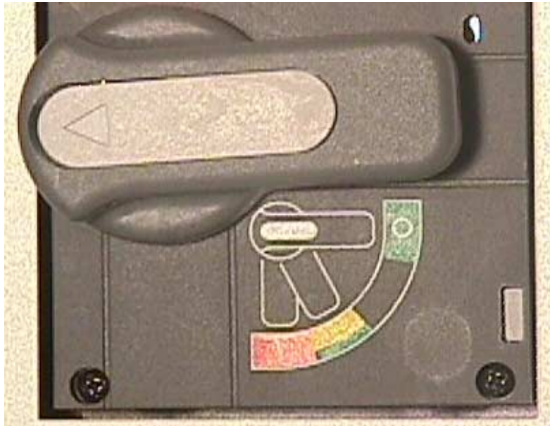
MAIN INPUT BREAKER IN THE OFF POSITION ILLUSTRATION 8-7
