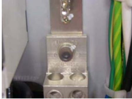
Figure 2-33 PDU System Ground Connection
