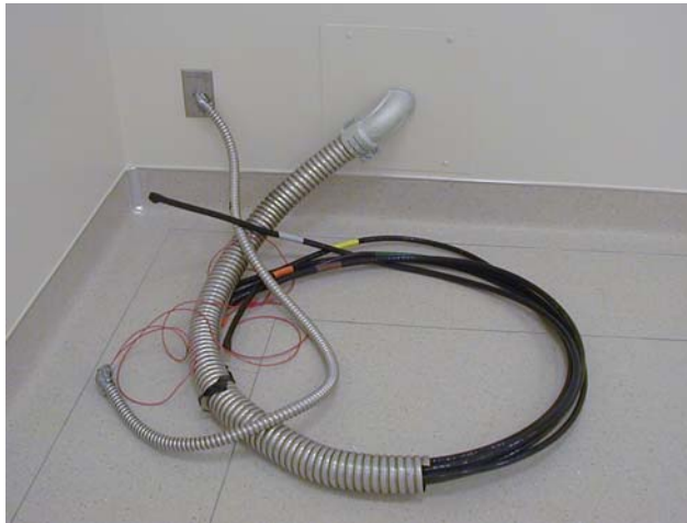
Figure 1-87 Flexible Conduit for PDU Power
