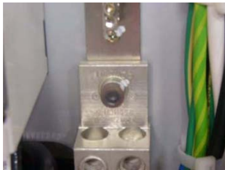
Figure 2-48 PDU System Ground Connection
