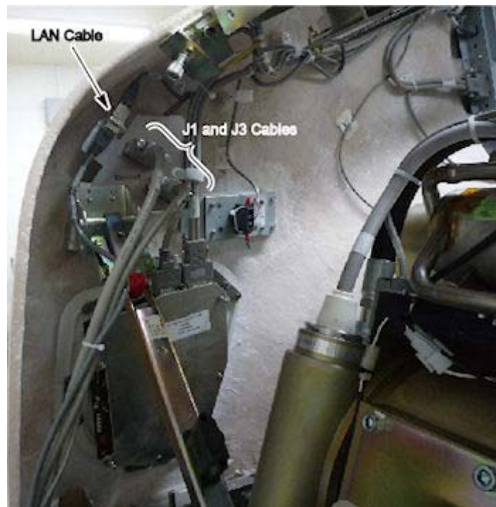
Figure A-13 Front Cover Cables
