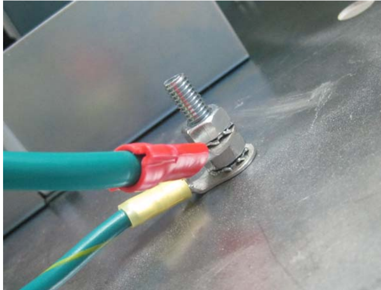
Figure 2-26 Ground Cable Connection
