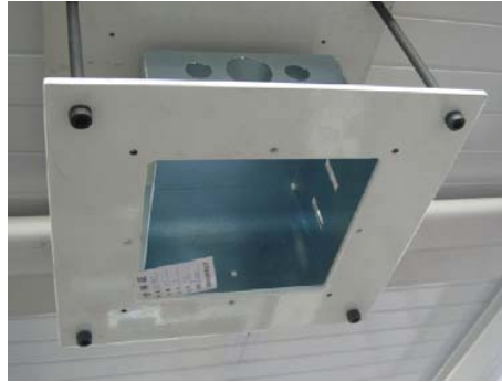
Junction Box Mounting Plate
