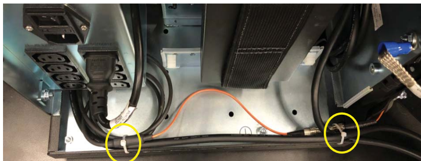
Figure 2-69 Route DVI Video Cables and Optical Fiber
