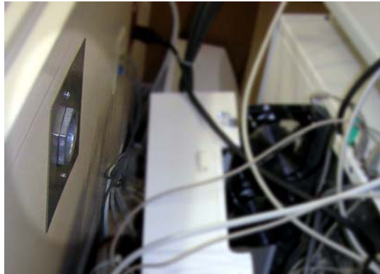
Figure 2-14 Wall Box (behind console)
