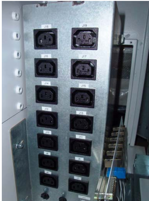
Figure 3-6 GOC6 Console power panel
