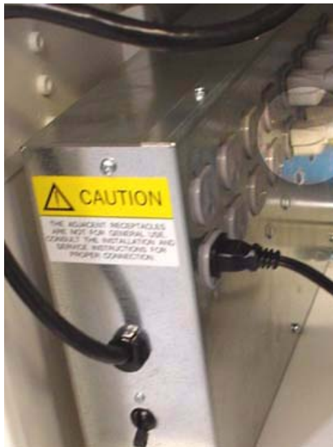
Figure 3-7 GOC5 Console power panel
