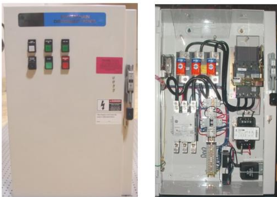
Illustration 18c: Typical OLD GE A1 MDP Front View & Interior View
