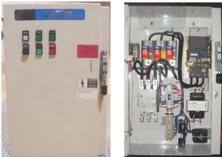
Illustration 11a: Typical A1 Panel Front View & Interior View.
