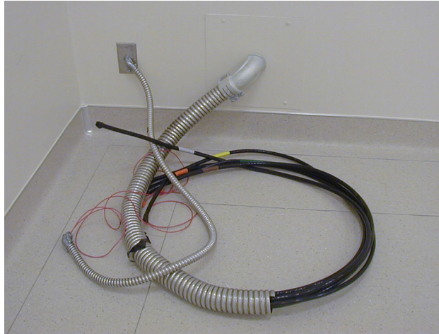
Figure 1-57 Flexible Conduit for PDU Power
