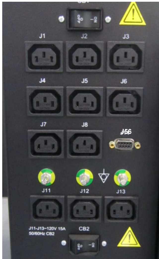
Figure 3-37 OpenOC AC Box Connections
