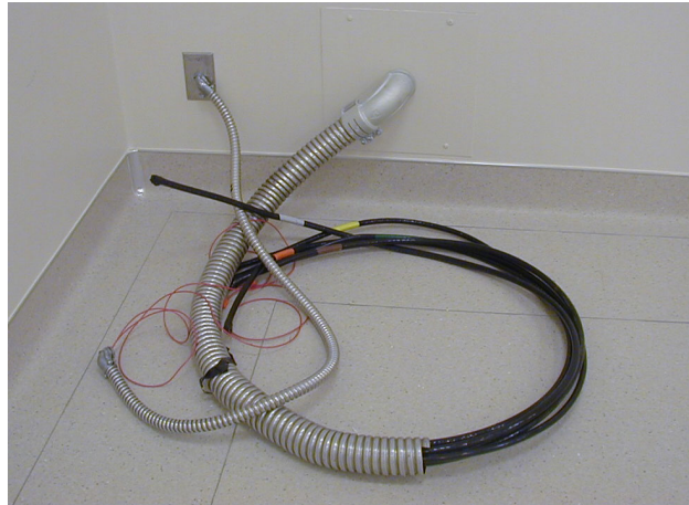
Figure 2-78 Flexible Conduit for PDU Power
