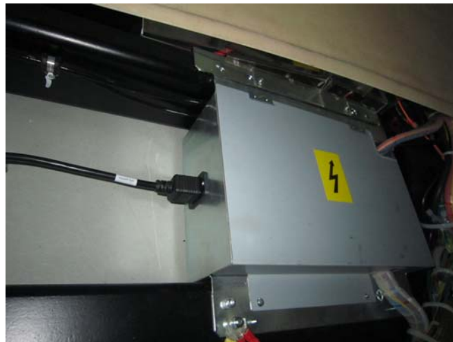
Figure 2-16 120VAC Power Pan
