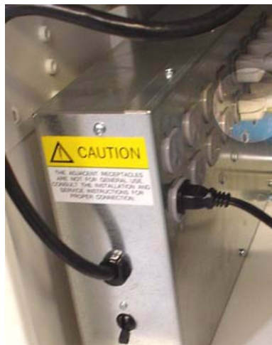
Figure 3-11 Console power panel
