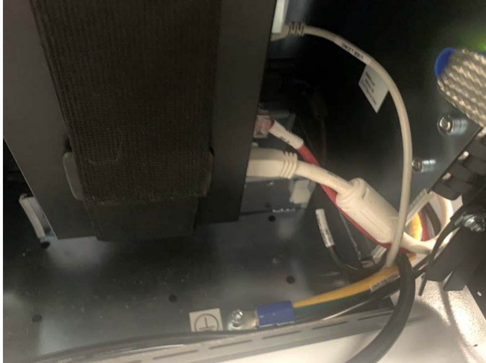
Figure 2-70 Ground Cable connect to Power Box
