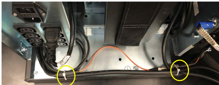
Figure 2-69 Route DVI Video Cables and Optical Fiber
