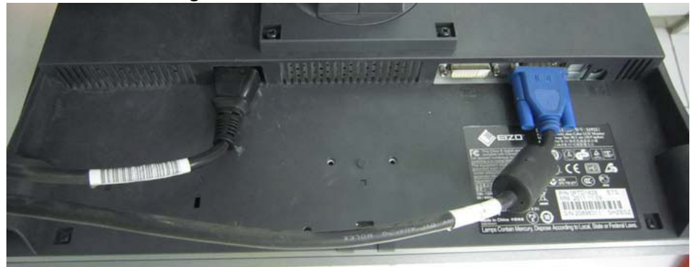
Figure 2-26 Video Cable and Power cable
