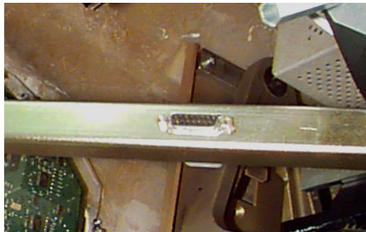
Figure A-17 Gantry Service Mode Cable Terminator
