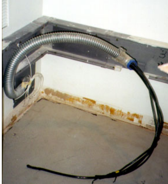
Figure 1-64 Flexible Conduit for PDU Power
