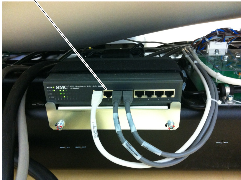
Figure 1-12 Cable Connection to LAN Switch
