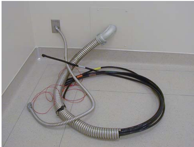
Figure 1-76 Flexible Conduit for PDU Power
