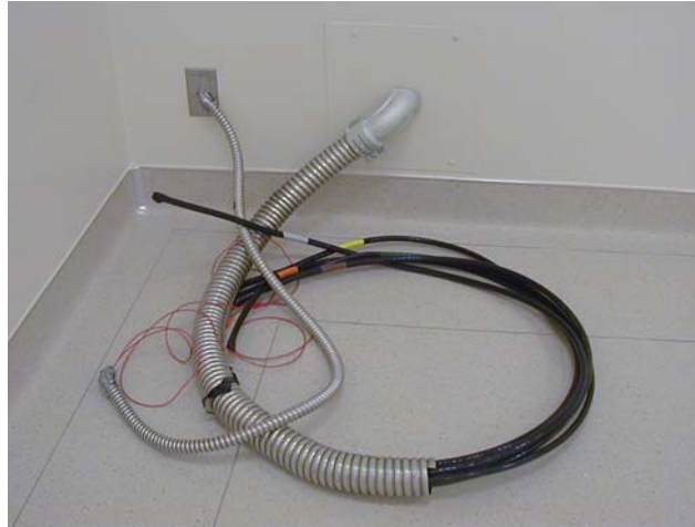
Figure 1-55 Flexible Conduit for PDU Power
