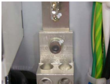
Figure 3-63 PDU System Ground Connection
