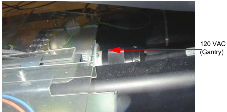
Figure 3-48 Gantry Power Pan
