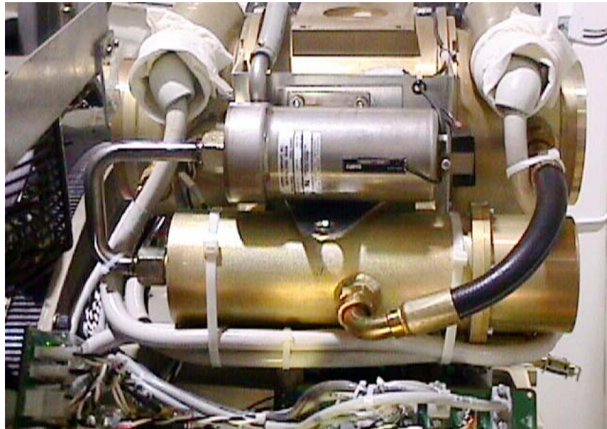
Figure 2-32 HV Cables Properly Routed and Secured
