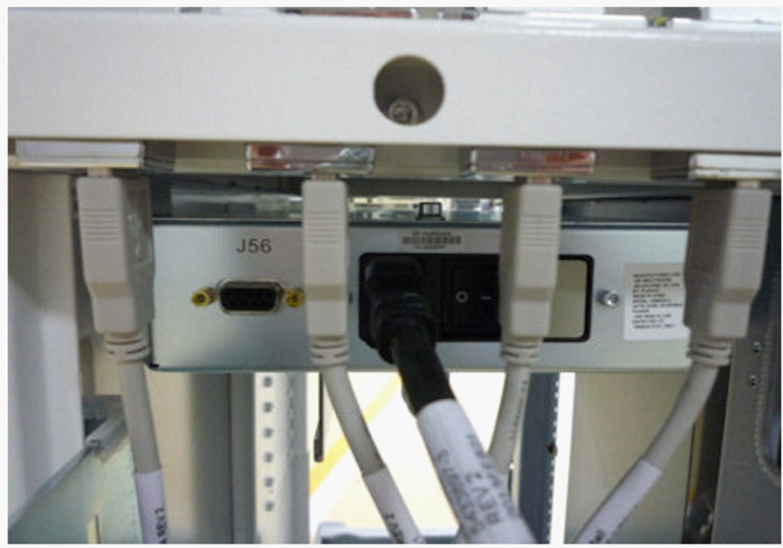
Figure 2-41 J56 Connector on Power Box
