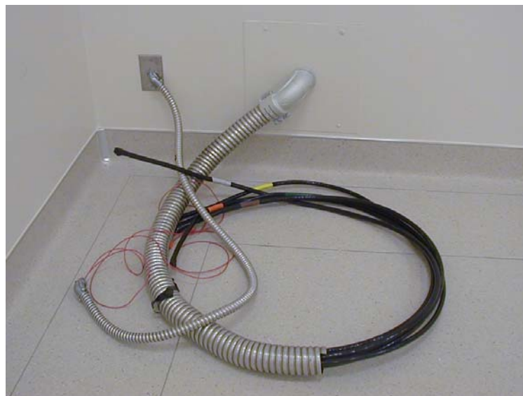
Figure 1-80 Flexible Conduit for PDU Power
